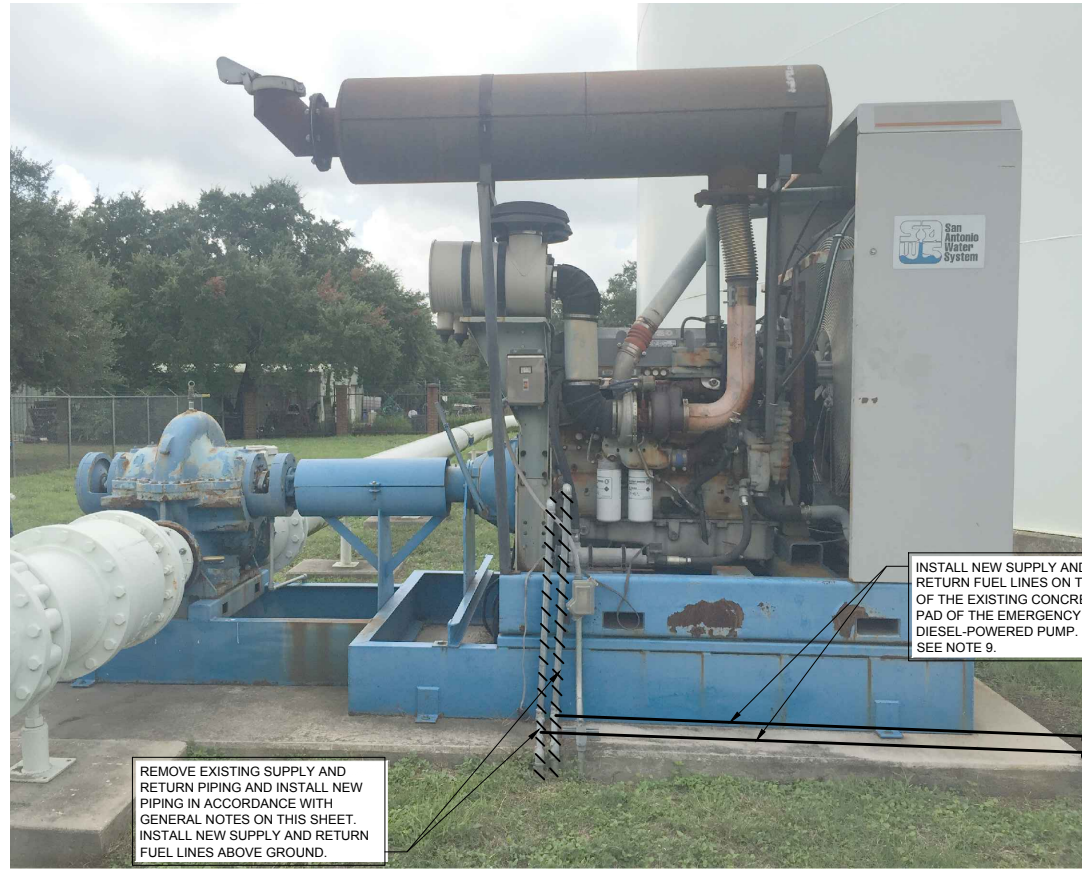
1 EMERGENCY DIESEL-POWERED PUMP C-02
