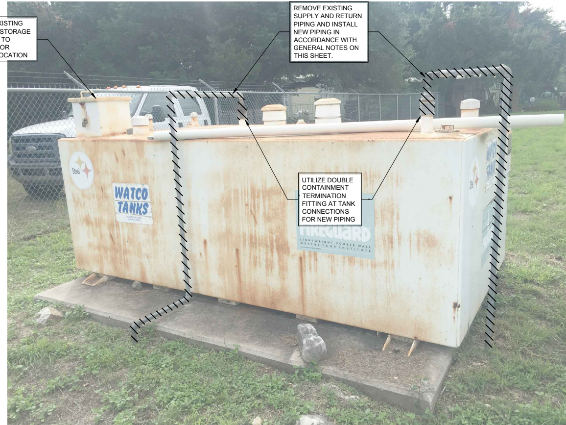
2 DIESEL FUEL STORAGE TANK C-02
